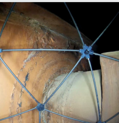
Corrosion and welds
